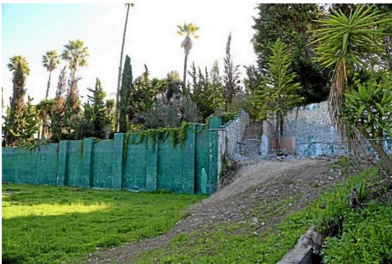
The retaining wall, athletic field were illegally build on parkland adjacent to the property of the Lugliani family. (Chuck Bennett / Staff Photographer)
